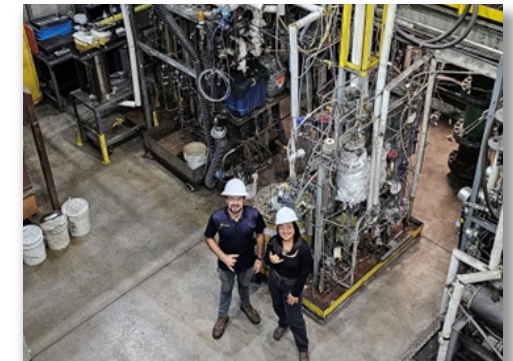
Gasification testing at Univ. North Dakota -
