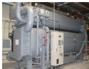
Greenhouse Cooling using Absorption Chillers
