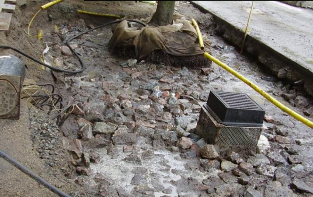
Ventilation chamber and inlet of surface water
